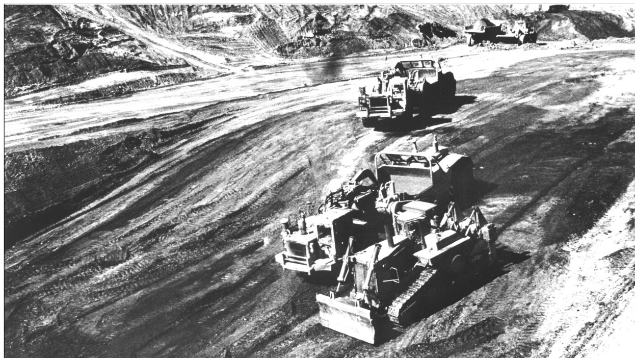
Figure 194. Initial scraper-dozer operations, Rasmussen Ridge Mine, date unknown. Photo by Peter Oberlindacher, BLM.
